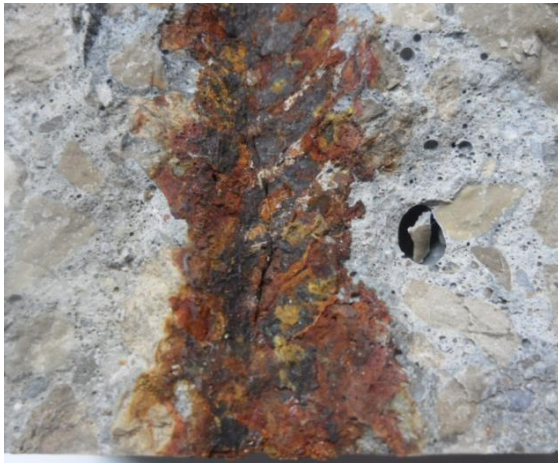
a) Corrosion signs on concrete
