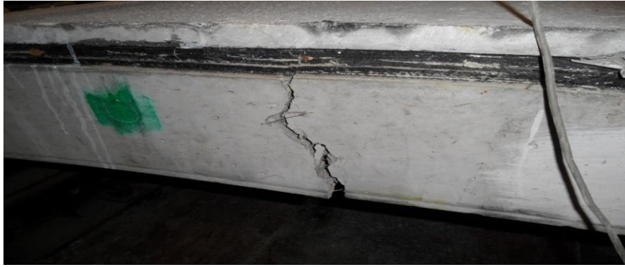
Figure .4– Cracking in SFRC lining segments.
