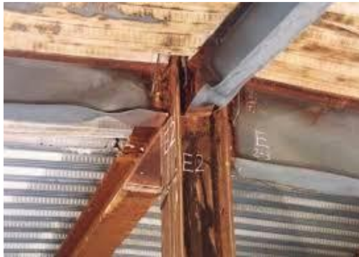
Fig.2.3 I beam Local failure
