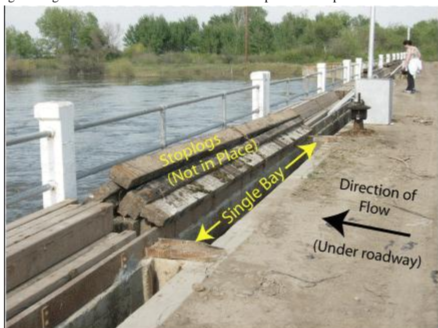
Fig: 1.1 Stop Log picture
